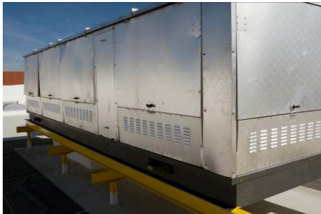
Integrated water-source refrigeration system
