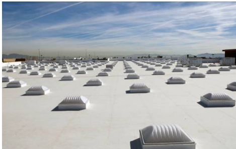
Skylights provide natural daylight
