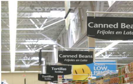
Store lights dim based on available daylight
