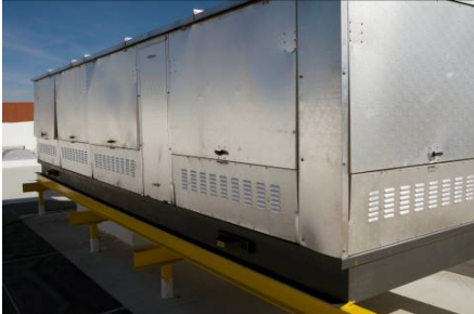
Integrated water-source refrigeration system
